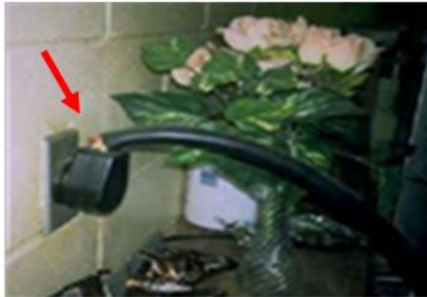
Cable has been pulled out of the plug end exposing internal wiring.
